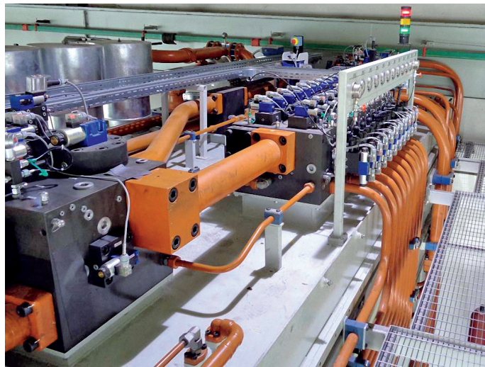
The hydraulic system for the 50-MN press
