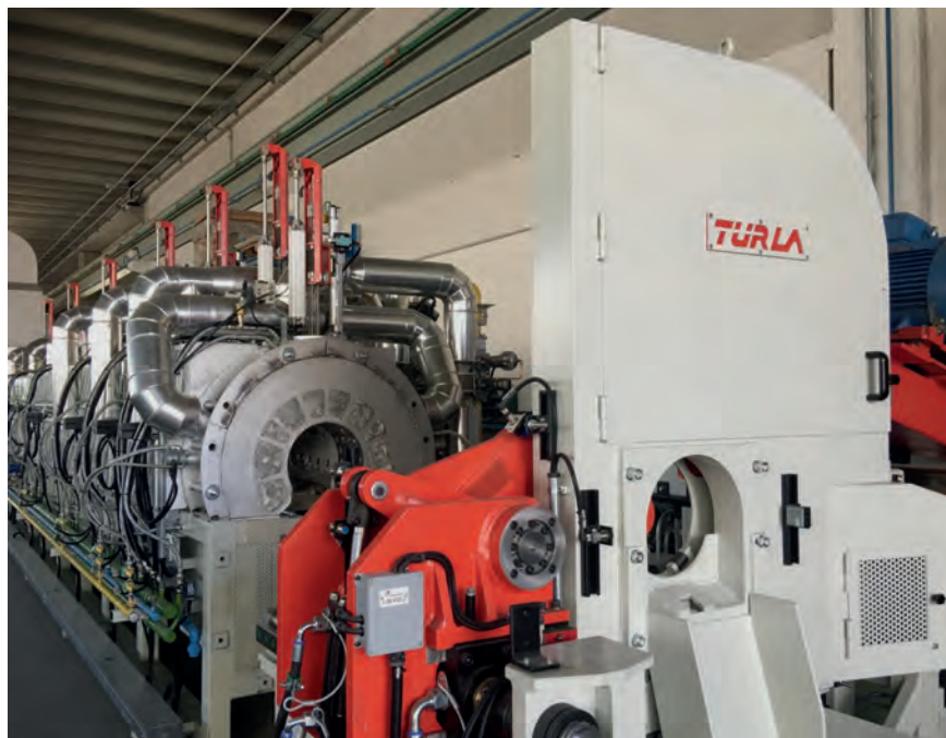
STeP5 Log gas heated furnace and hot log saw
